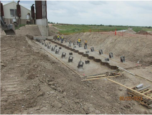
Fully prepared western floodwall foundation with 34 H piles set 25 ft deep with sheet piling down 30 ft. 5/2/2023
