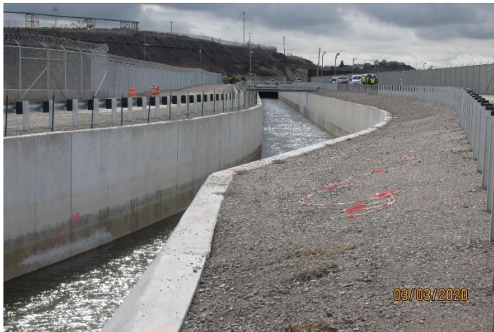
Looking downstream in Upper Reach along new rectangular section. End of Upper Reach at closed culvert.
