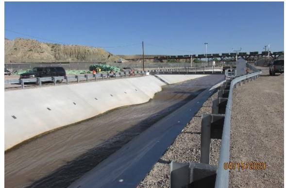
Hydraulic jump caused by Parshall Flume for gaging 4/15/2020
