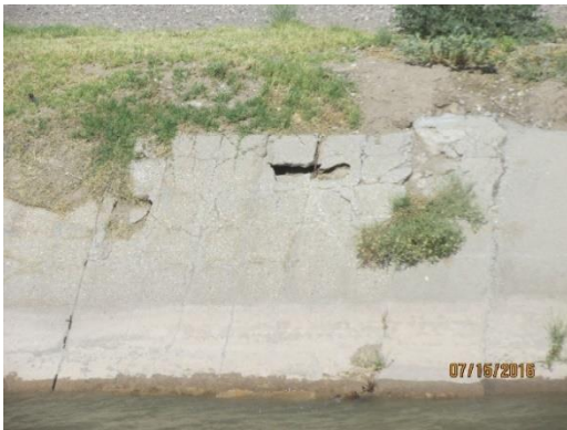
Average condition of Upper Reach prior to rebuilding 7/16/2016
