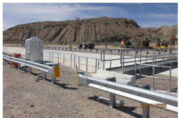
New Water Accounting (gaging) area and bridge 3/31/2020
