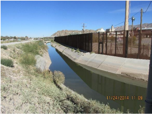
Looking upstream from approx. Sta 106+00. Note damaged concrete panels. 11/24/2014
