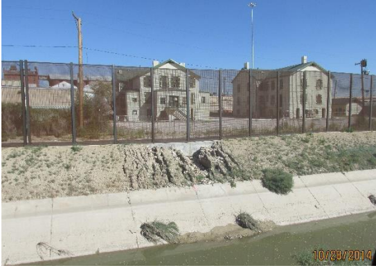
Example of erosion that occurs between the DHS fence and the canal. 10/28/2014
