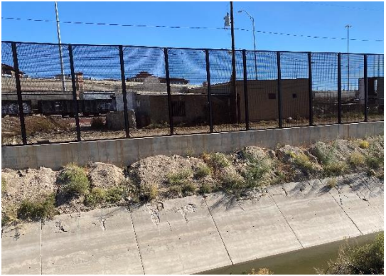
Example of erosion and existing concrete damage 11/29/2022
